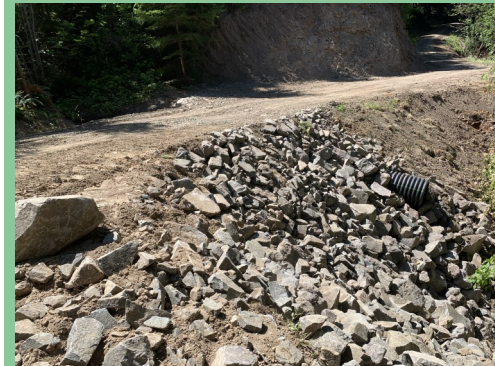
Sierra Pacific Industries employs a variety of sediment control measures to protect water quality in its road building and crossing installation operations, including liberal use of well placed rip rap (Oregon District).
